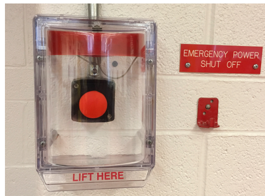
Figure 7 Emergency Power Shut Off Button
